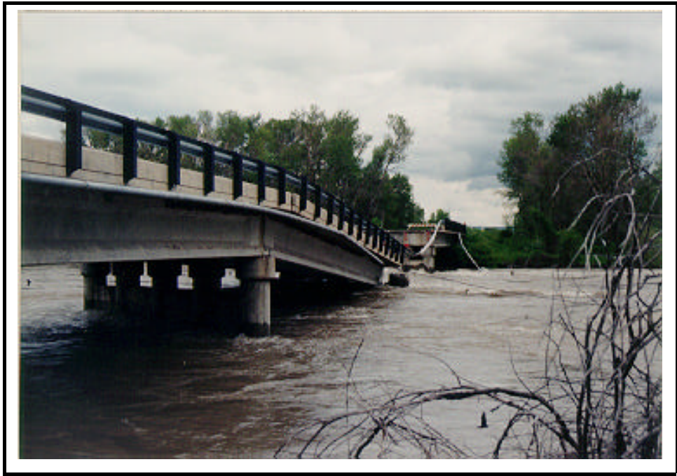
Archer Highway bridge across the Snake River between Ririe and Rexburg, Idaho.
