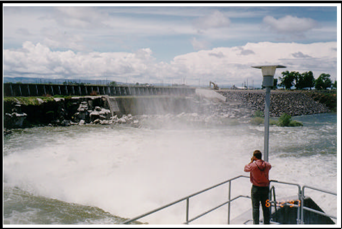
MilnerDam stilling basin sill and downstream river section with the old spillway in the background. The at-site powerplant, which typically provides required minimum instream flow in the one mile down to the powerhouse, is in lower right of picture. The project is currently spilling about 17.5 kcfs.
