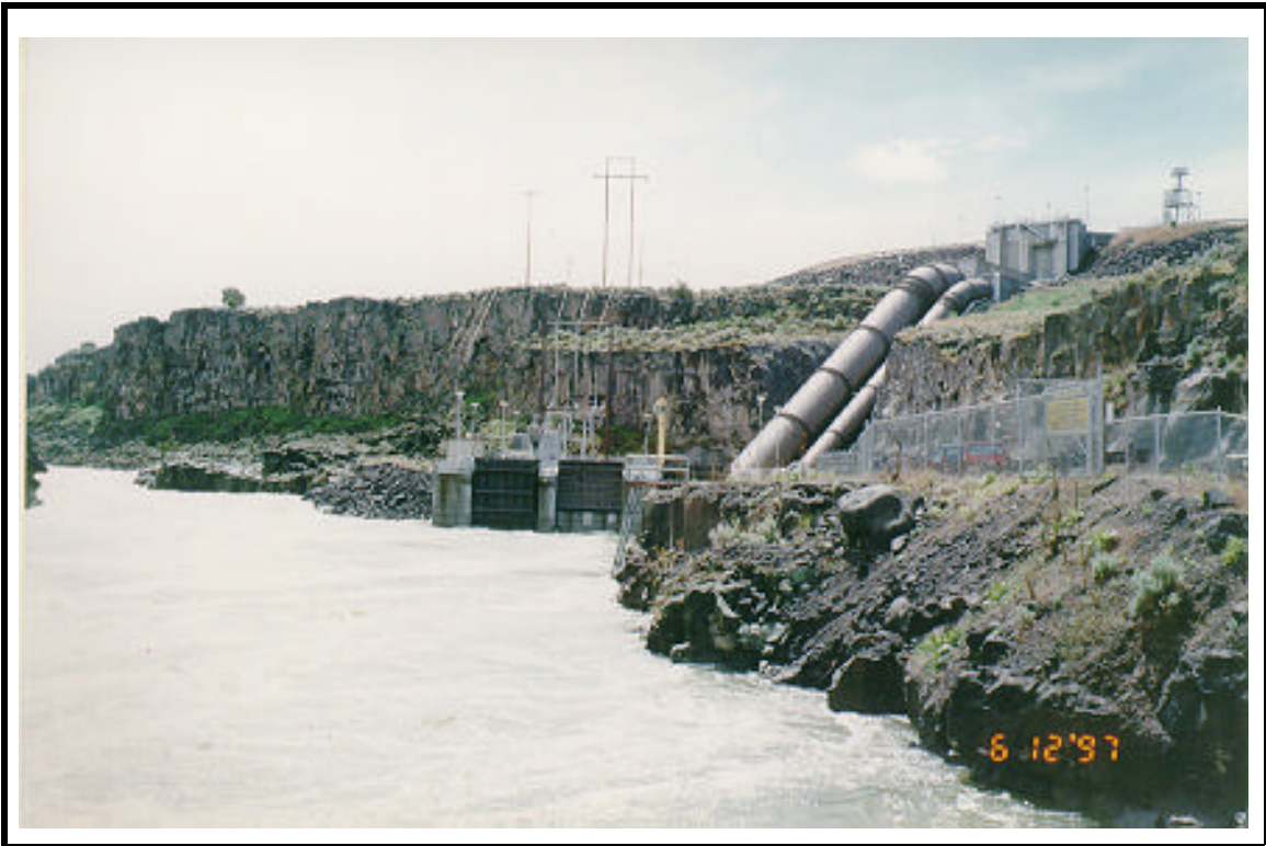
Milner Downstream Powerhouse. The Southside canal carries 8500 cfs from the Milner pool to feed the south side canal irrigators and the Milner downstream powerhouse, which has a capacity of 5.5 kcf and 58.5 MW from the two units. Powerhouse inflow is controlled by the structure pictured above.
