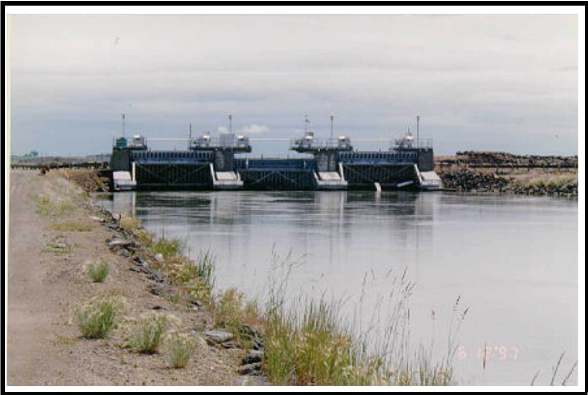
Control structure on southside canal (one mile below Milner) controls both the flow into the downstream powerhouse, which is located just upstream and to the left of this structure, and the irrigation flow in the canal.
