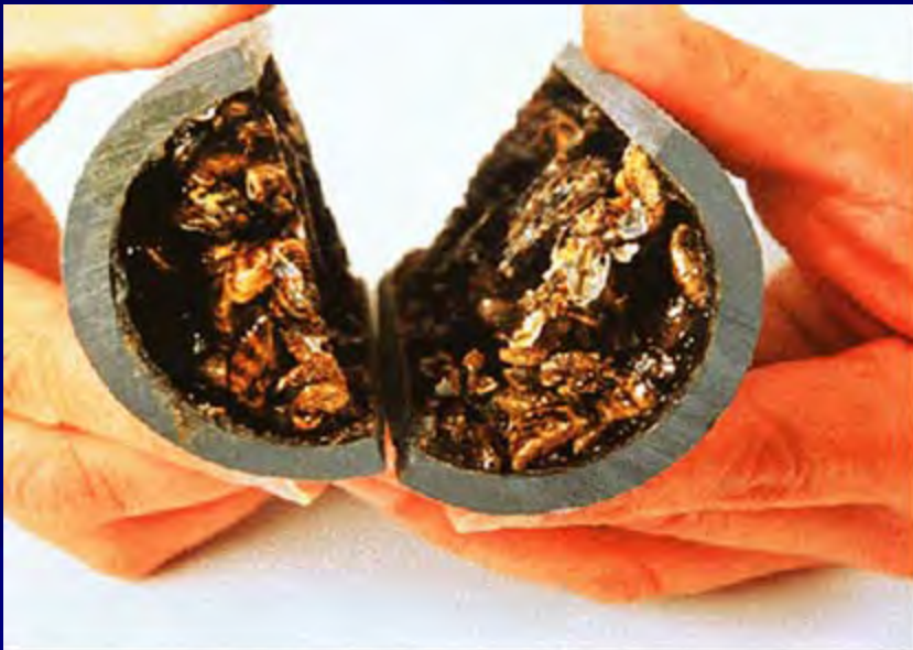
Pipe clogged by one year's growth of zebra mussel
