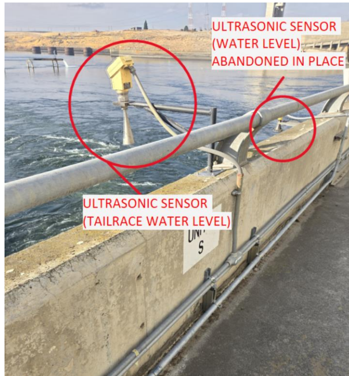
Figure 5: Tail Water Level Sensors
