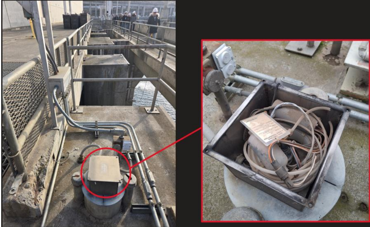
Figure 10: Stilling Well – Water level Sensor Metritape
