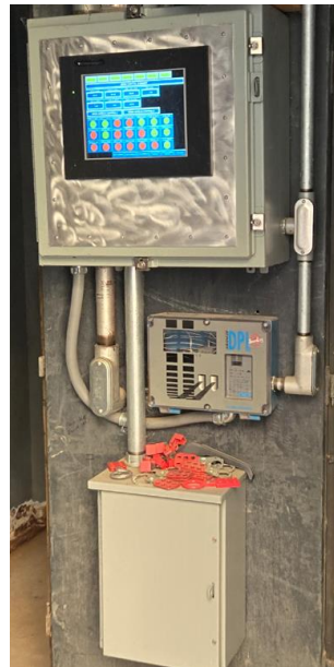
Figure 14: North Fishway HMI/PLC Cabinet In FCQ4 Shack
