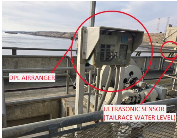
Figure 8: Central Weir Gate Sensor & Devices
