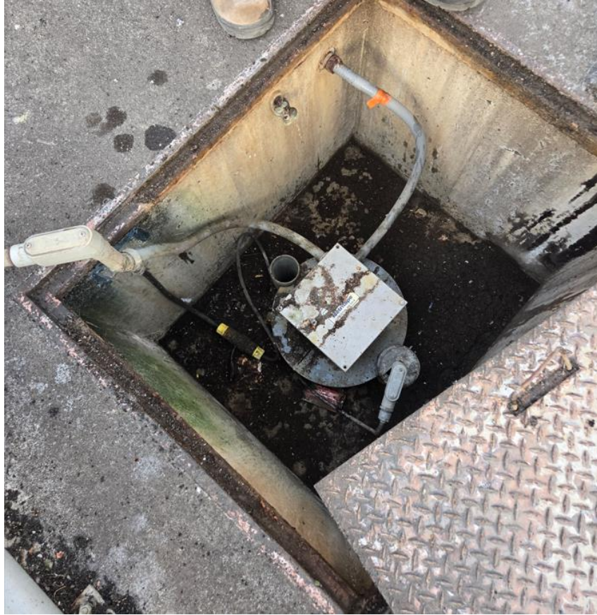
Figure 13: Stilling Well – Water level Sensor Metritape
