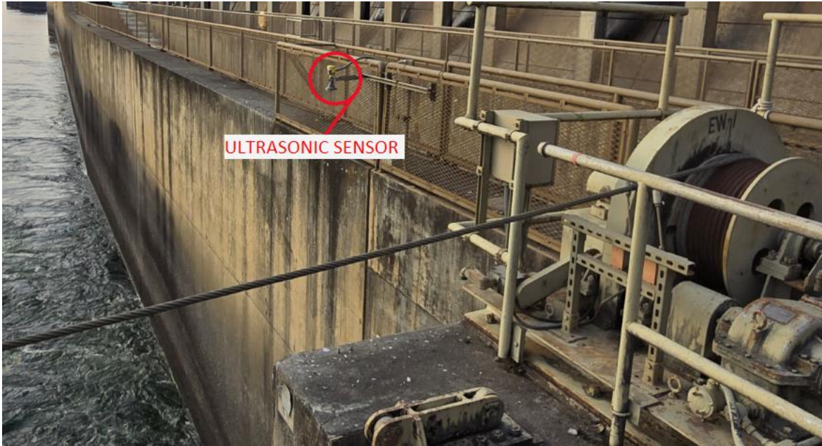
Figure 11: North Fishway Tailrace Ultrasonic Sensor
