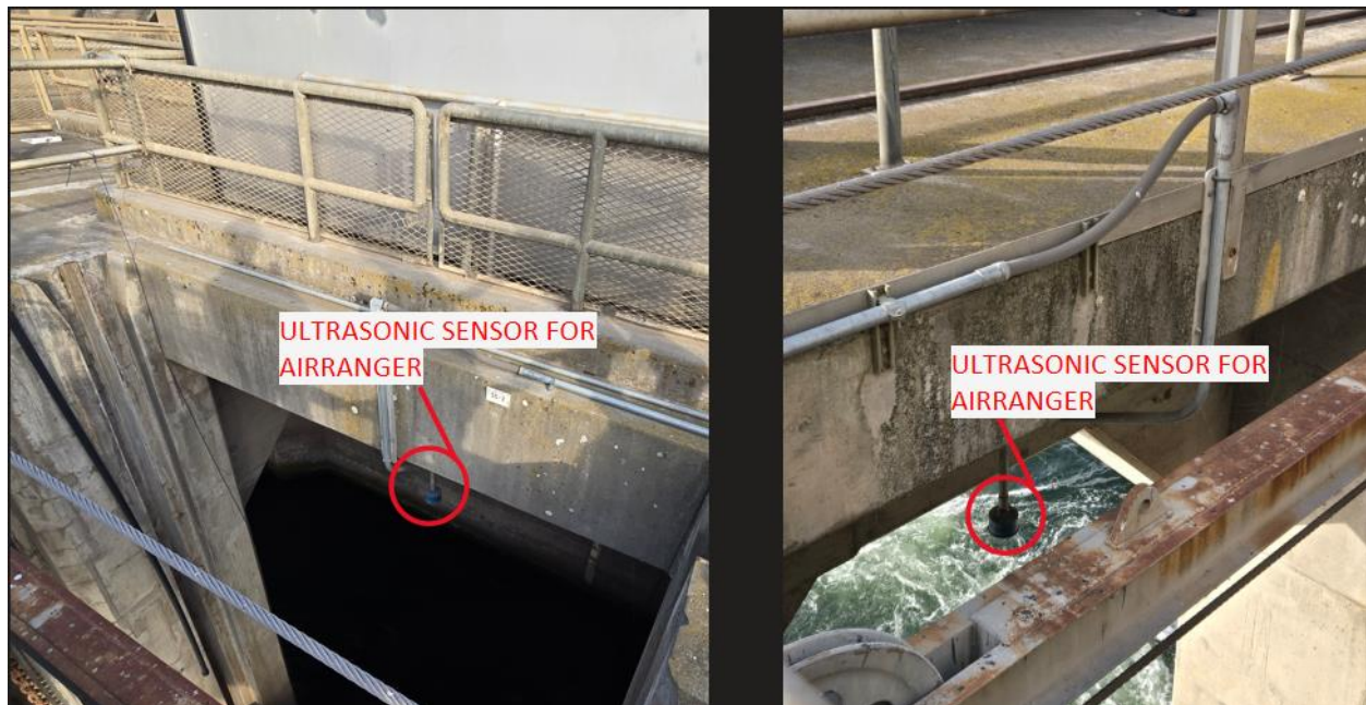
Figure 9: Central Weir Gate Ultrasonic Sensors
