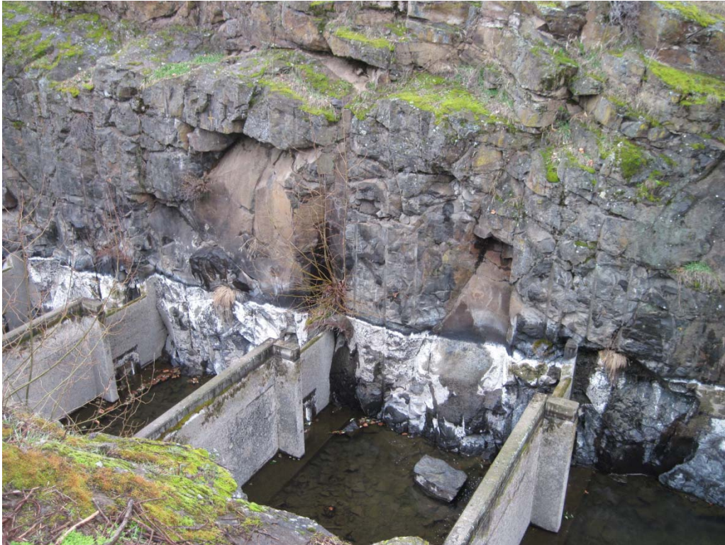
Photo 2 - Showing areas of recent rock block fall. Localized rock anchors are required.
