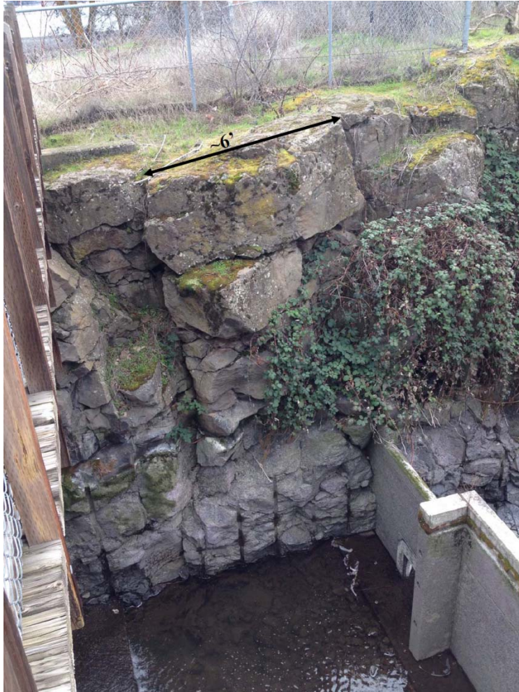
Figure 11 – Photograph looking south towards the southern fish ladder rock cut near weir 130. Rock blocks up to 6 feet in diameter have weathered out of the cut face in this area.
