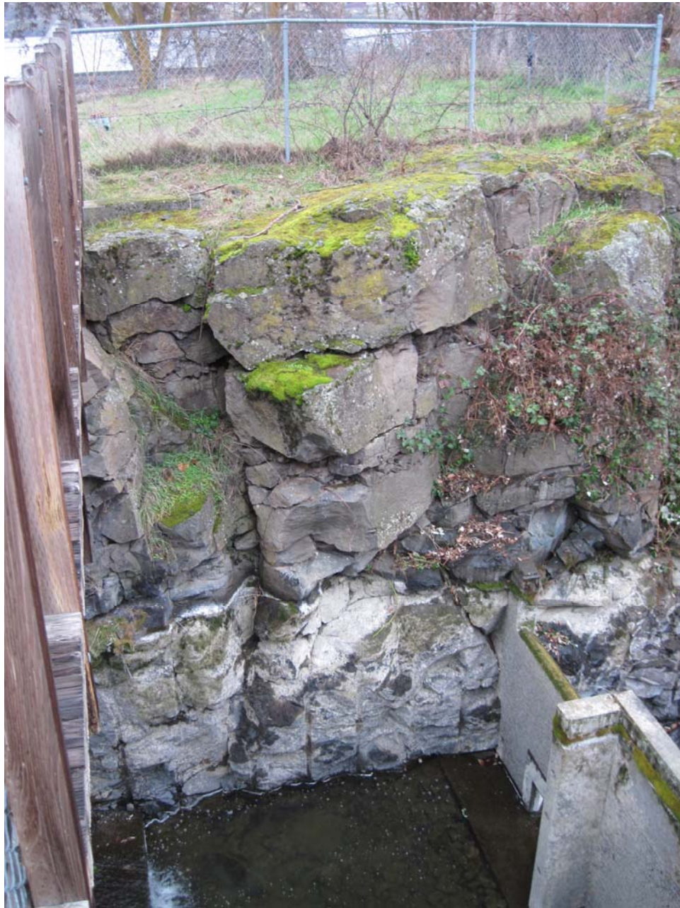
Photo 8 – Area of unstable rock blocks, near footbridge. Although these blocks appear unstable, it would be difficult to anchor or scale this area without threatening damage to the fish ladder. This area should be monitored, and any work in the area should be done to limit impacts to the slope. Workers access to this area should be limited.
