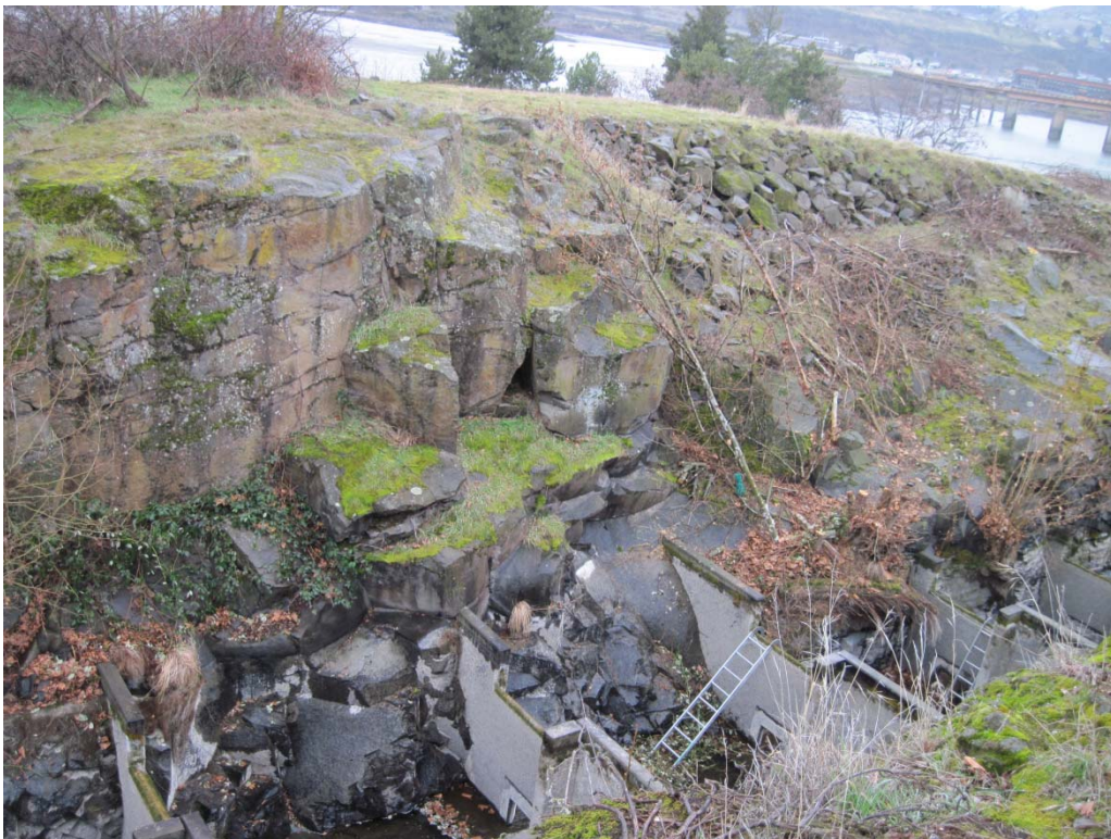
Photo 3 – Showing large rock blocks that may be at risk of toppling. Localized rock anchors may be required.
