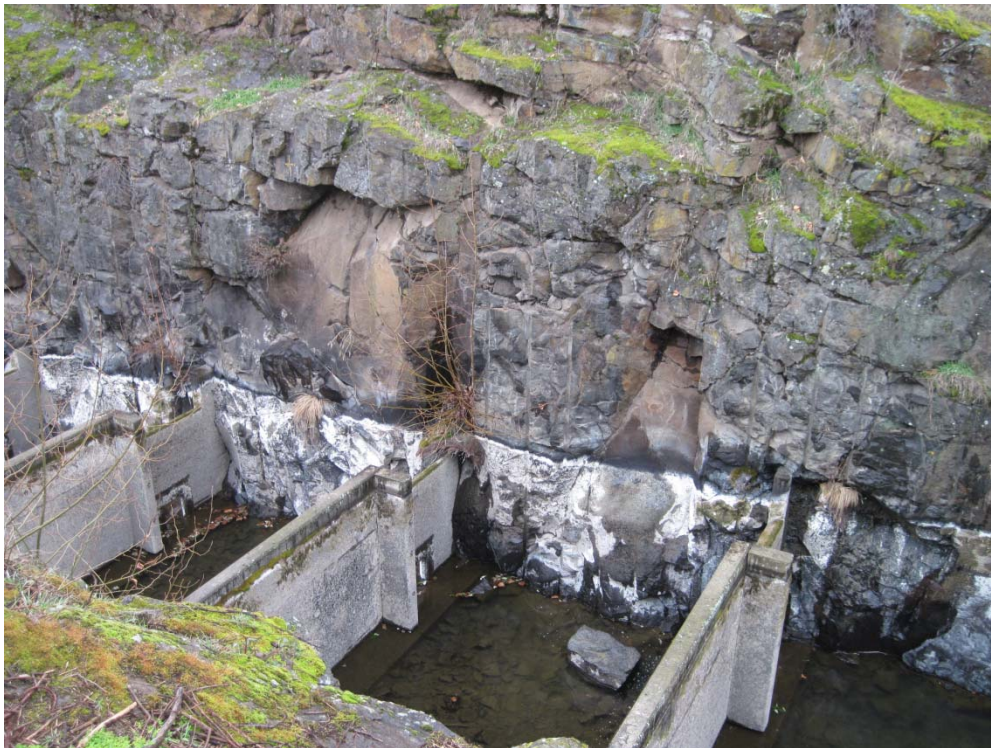
Figure 13 – Photograph looking west towards the northern part of the fish ladder, showing recent rock fall.
