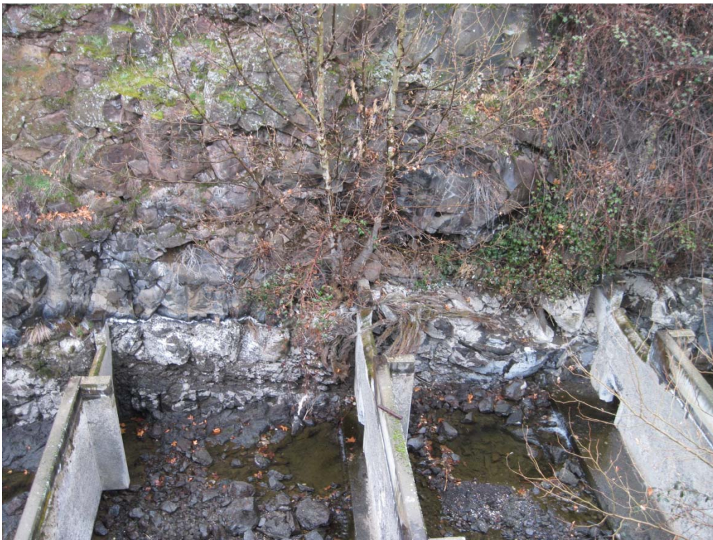
Photos 4 & 5 – Sections of rock cut needing vegetation removal and scaling.
