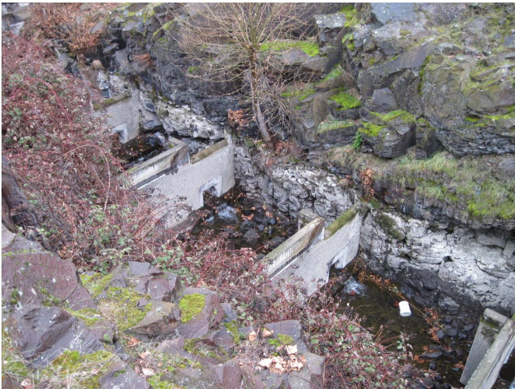
Photos 6 & 7 – Area of lower rock cut being eroded and undermined by water flow. This area of cut may require construction of a concrete wall structure to protect lower rock cut for further erosion.
