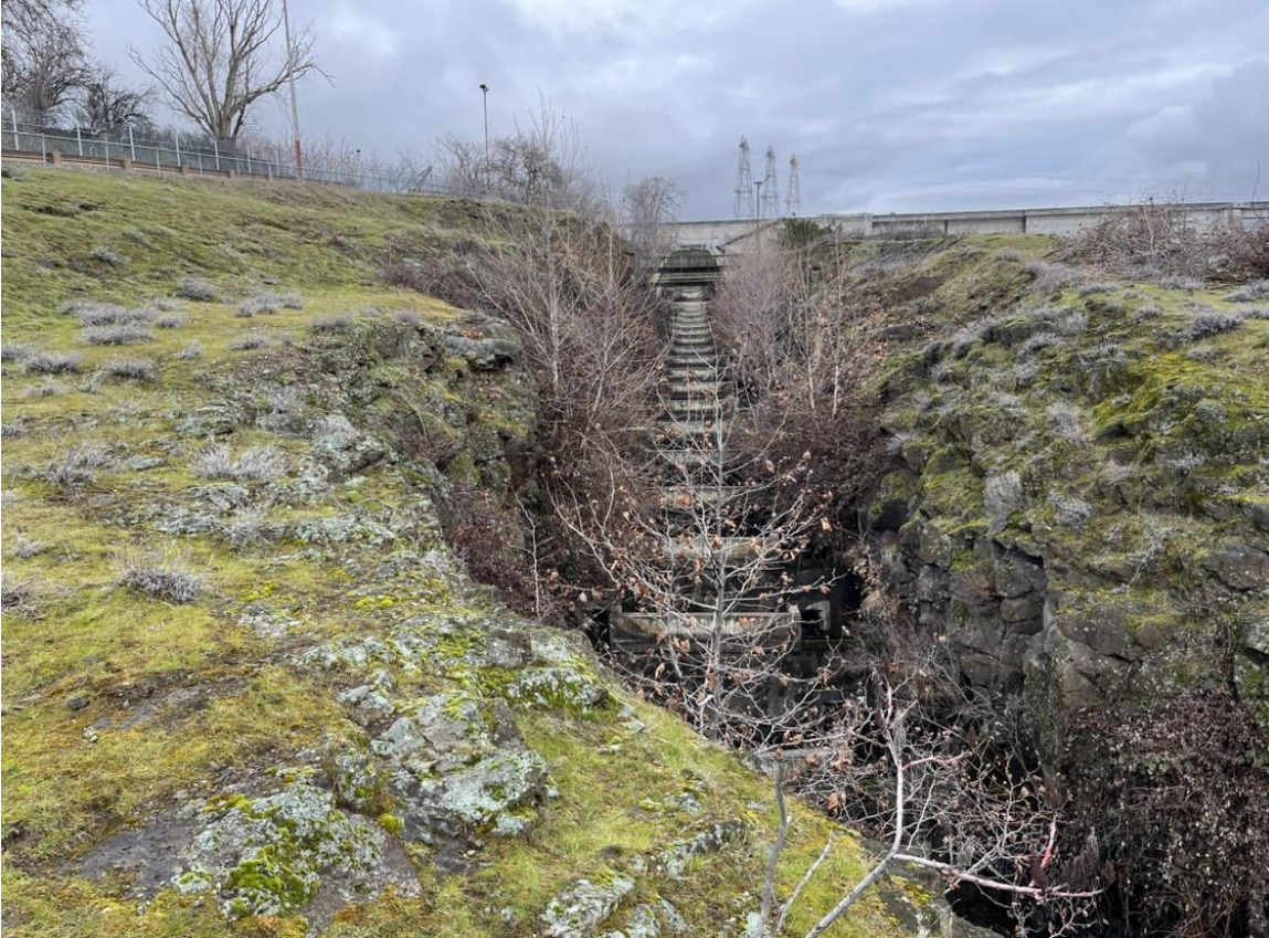
Photo 1: Looking northeast from west bend of north fish ladder, looking at north half of the ladder.
