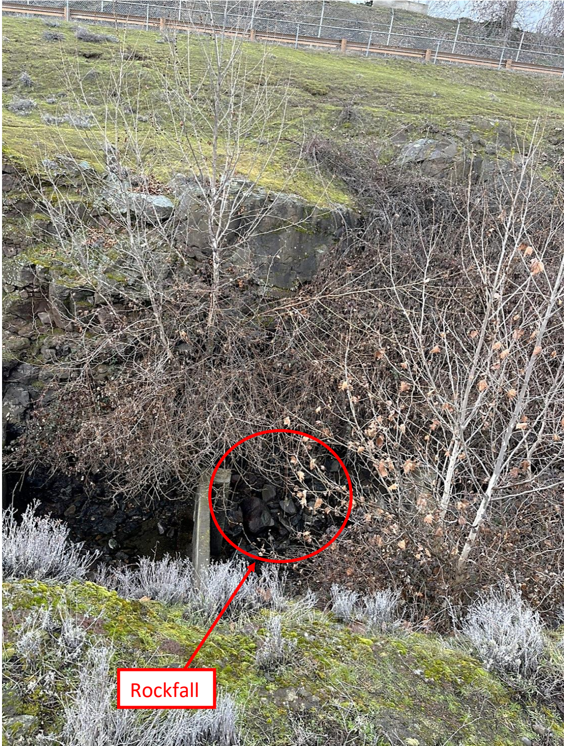
Photo 4: North half of north fish ladder, looking north and down into fish ladder at Weir 116 and adjacent rockfall
