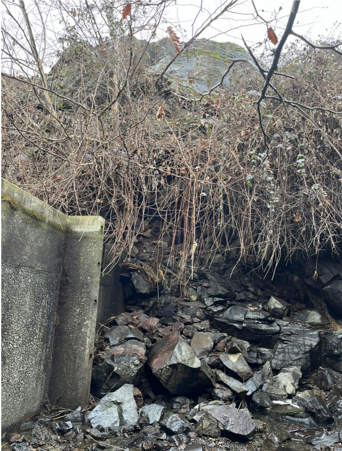
Photo 6: Rockfall adjacent (east side and north end, south-facing wall) to Weir 116. Larger rock pieces blocking weir opening (opening is not visible due to blockage). Heavy vegetation and overhanging rock mass shown at top of photo.
