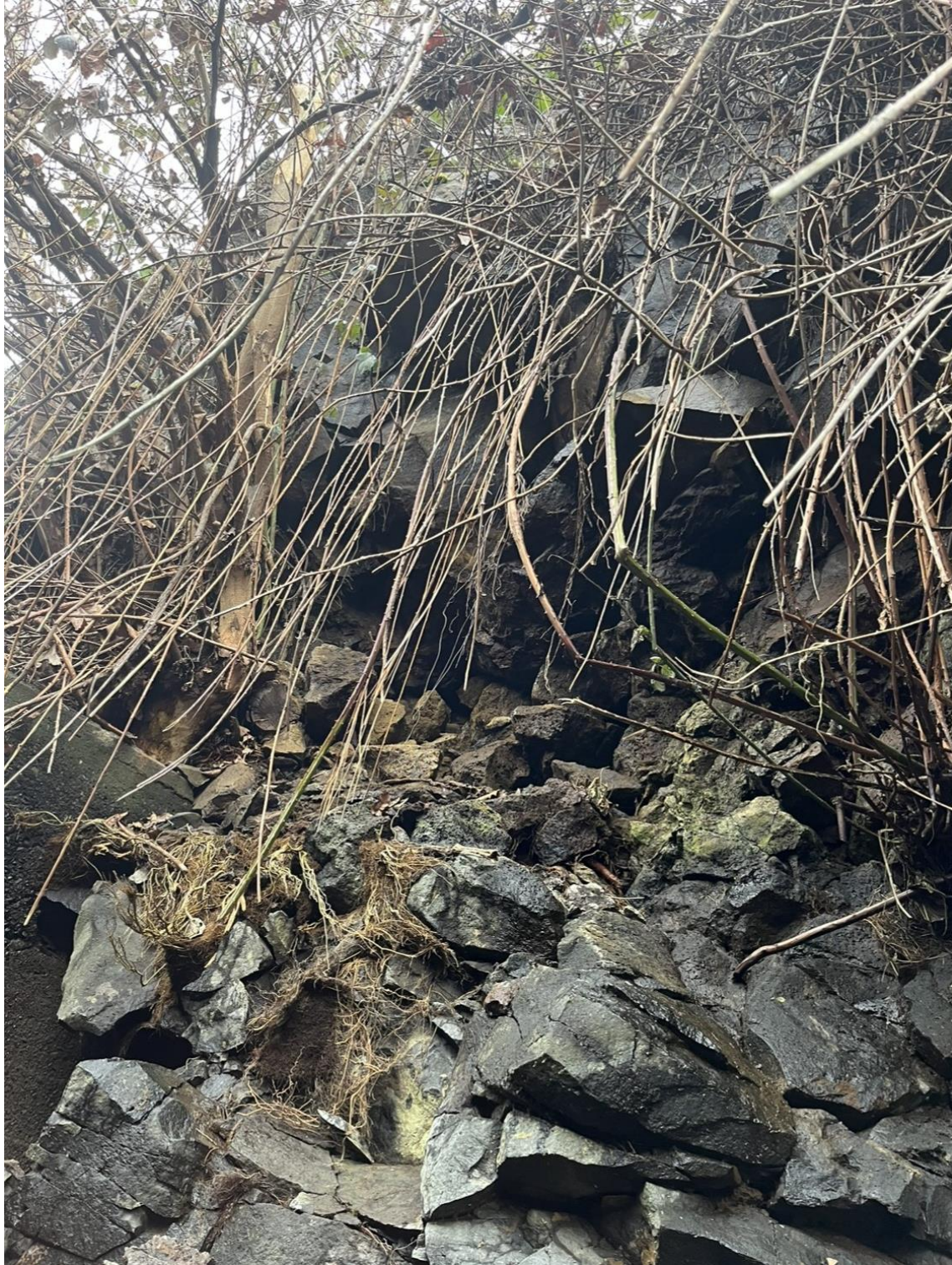
Photo 8: Close-up of pocket left from rockfall, overhanging rock mass, and tree root system near top and north end of Weir 116, north fish ladder.
