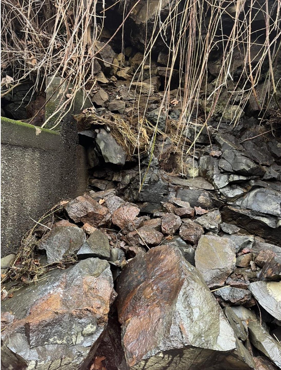
Photo 7: Close-up view of rockfall pile, north fish ladder, south-facing wall, east side/north end of Weir 116.
