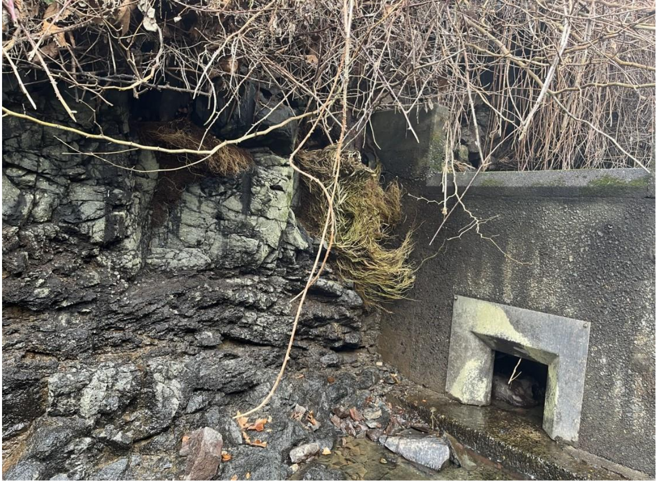
Photo 5: Interior of north fish ladder, looking at north end and west side of Weir 116, south-facing wall. Weir opening shown is opposite side of rockfall blockage. Rockfall boulder visible through opening.
