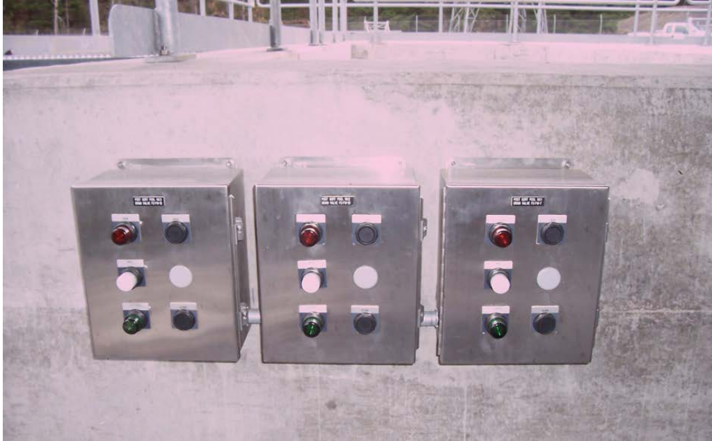
Figure 14 –Controls for Drain Valves for Sorting Pools
