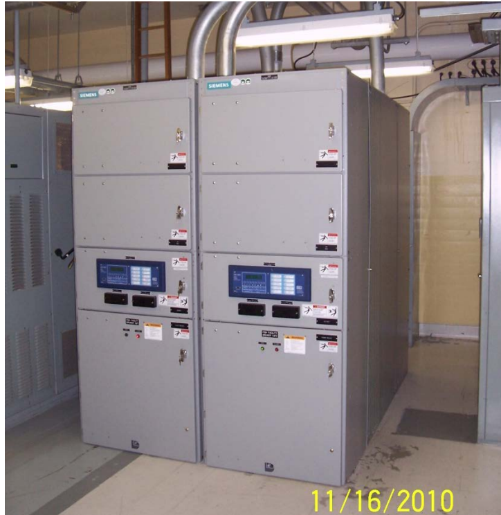
Figure 11 – Primary Feeder Breakers
