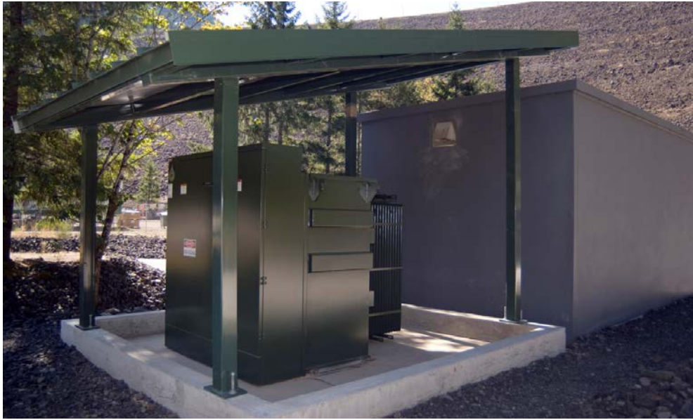
Figure 12 – Pad Mounted Transformer
