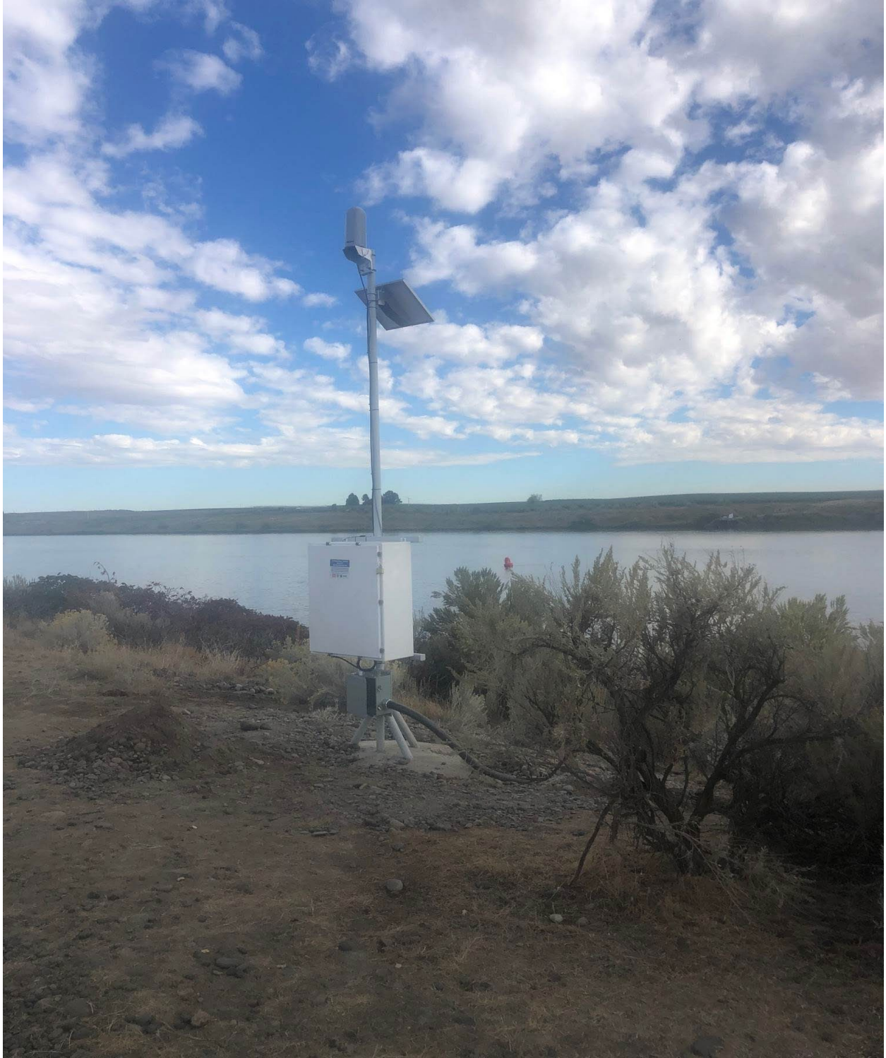
Figure F-12. New mast, NEMA box, solar panel, and antenna installed at IDSW.
